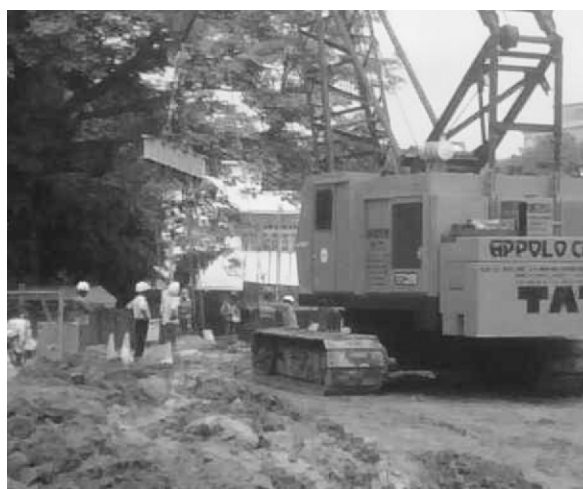
Construction Site in Maharashtra. Large Numbers of Migrant Men in India are Employed Under Contract System.
